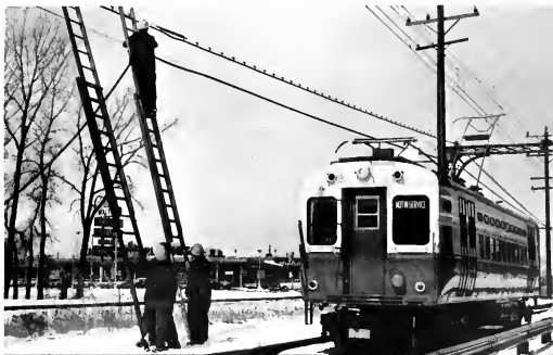
Signal, communication and station lighting cables were being installed while the first test run of car #1 through to Dempster was being made on March 30, 1964.
